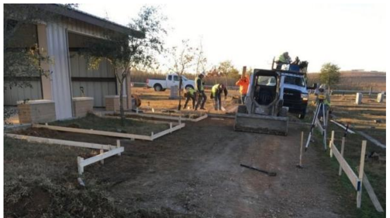
Danny Smith worked with his Chandler Concrete crew to pour a parking pad and sidewalks at the St. Peter's Cemetery pavilion. They also made concrete pads for the new granite benches that will be installed around the cemetery soon. Photo courtesy Dana and Danny Smith.
